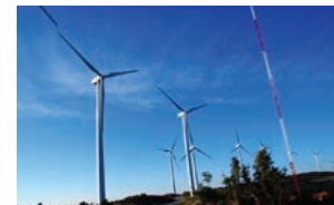
Wind Farm Monitoring (SCADA)
